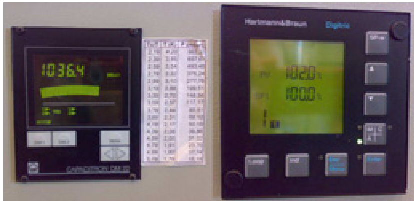
Figure 5.9: The cryostat pumping line control panels.
